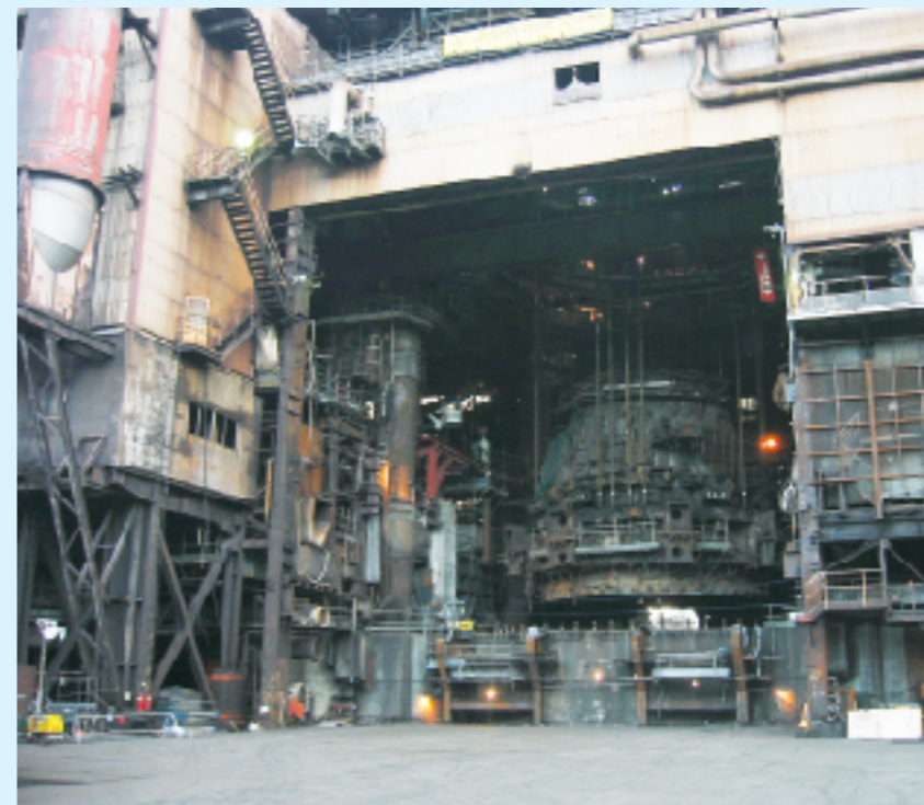
Blast furnace at JFE Steel's Kurasiki Works (lifting weight: 4,500 tons)
