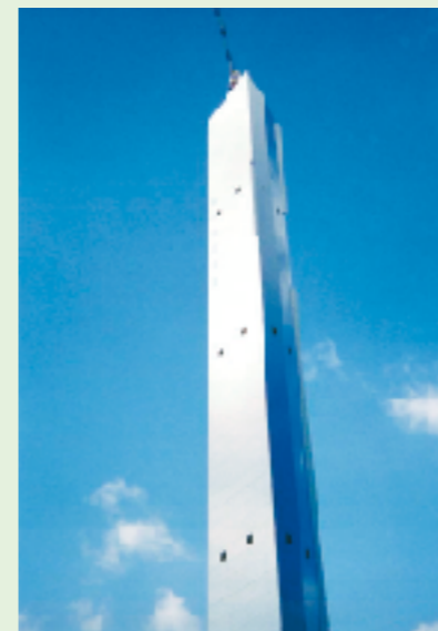
Jump-up method for stuck at waste incineration plant of Tokyo Chuo Area
