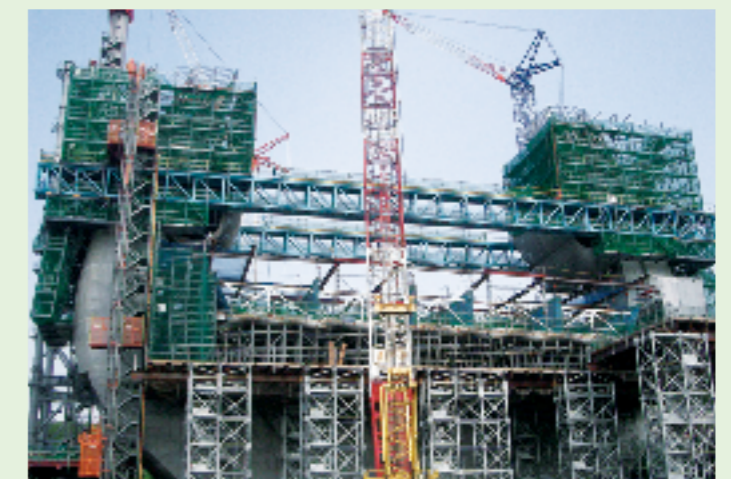
Climbing scaffolding method for main tower for Yahagi River cable-stayed bridge at Second Tomei Expressway
