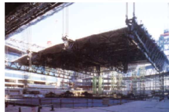
Lift up of large roof at Saitama Super Arena (lifting weight: 3,540 tons)
