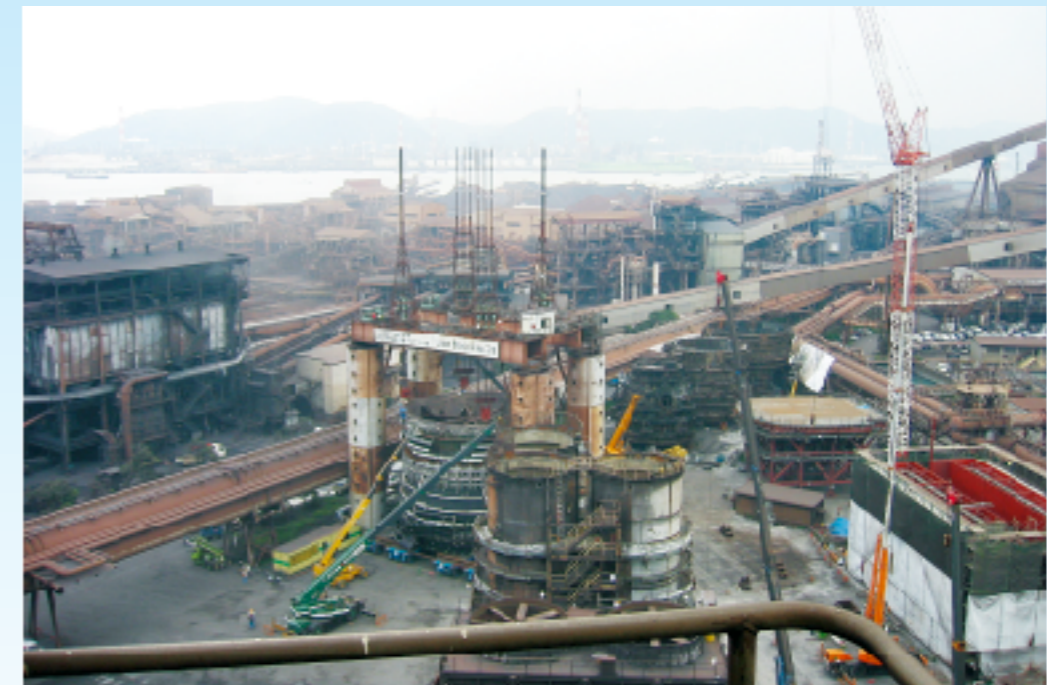
Up & Down Method used in relining of No. 2 blast furnace at JFE Steel's Kurasaki Works
